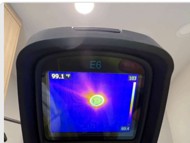
Air infiltration around flush-mount LED light fixtures above laundry room (note conditioned space above—possible air infiltration into/through framed floor assembly)
