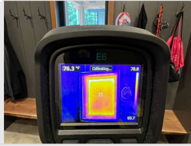
No air infiltration around window trim
