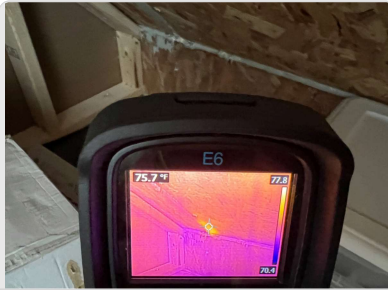
Minor air infiltration around seam between SIPs roof and wall in attic/knee wall space over garage
