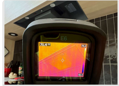
No air infiltration around range hood
