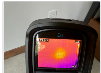
Minor air infiltration around exterior wall electrical boxes
