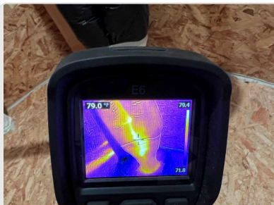
Air infiltration around ERV intake/exhaust penetrations to outside
