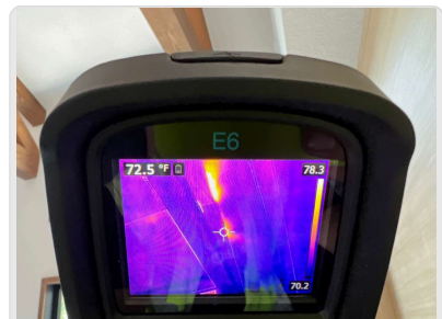
Air infiltration around vaulted ceiling beam above kitchen
